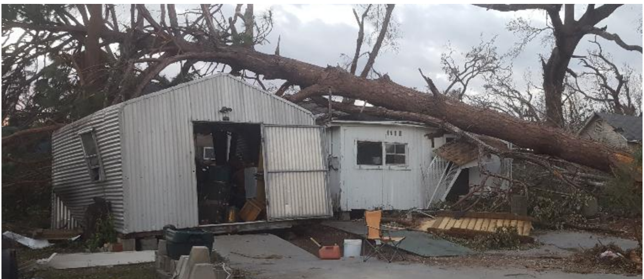
The smallest rental, only 500 sq ft. Power head and box ripped off by tree. Bamboo helped it from being worse maybe by absorbing some of the wind. That's a pecan tree lying on the roof, my granddad planted that back in the 1960's. His shed in back has a blue tarp, so must have gotten damaged. He built that just last year, 8x12'.
